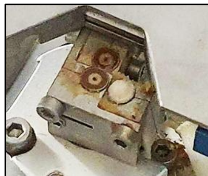
Pic 2. Flux residue at spray head; crystallization of solids due to a leak
